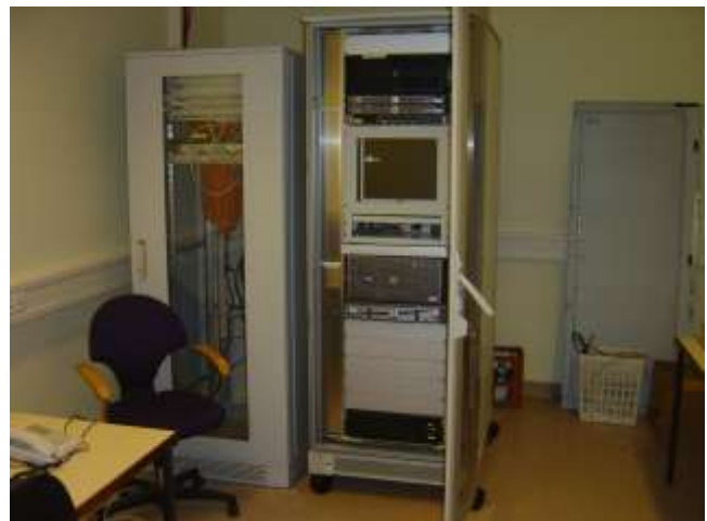
New Server room with VEPRO 3TB Power Server
